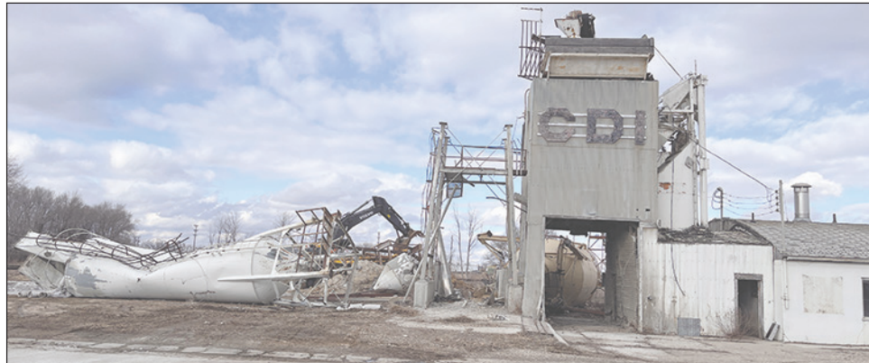
The old CDI Ready Mix building, located at the corner of the 500 block of Fir Avenue, is being torn down. Jay Harris said it's a safety hazard and he's bringing it down.
